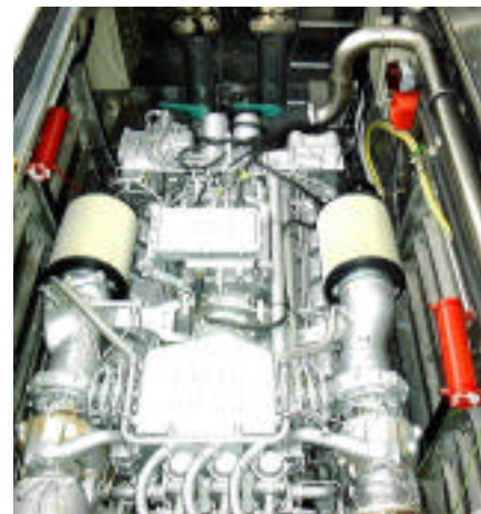
Marine installation in a high-speed power boat
