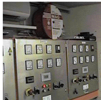
In addition to protecting the entire sub-station control room, as shown, smaller MAGs can be mounted inside the control cubicles to provide local protection
