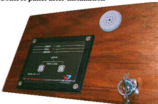
Sounder at top corner and ignition switch in lower right corner.
